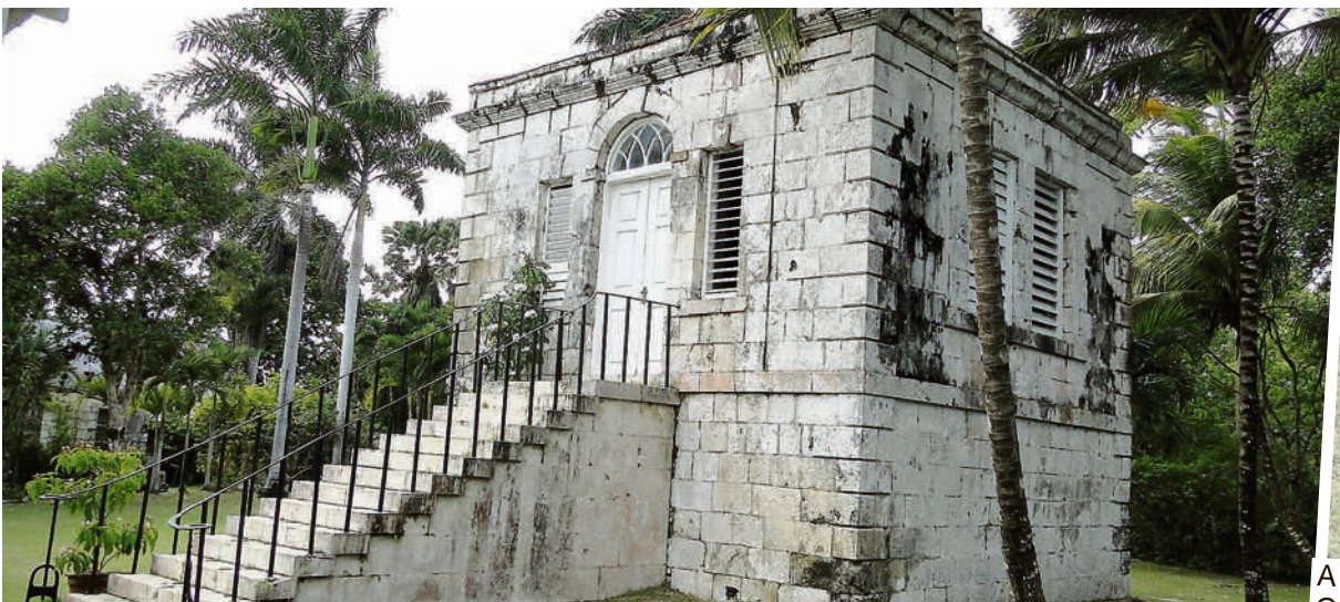
The counting house, where the financial matters of Good Hope Estate in Trelawny were controlled.
